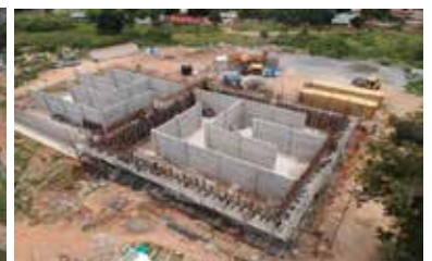
Reservoir 5000 cum Capacity Located at Tabora
