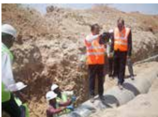
Pipe welding checking by using ultrasonic test during the inspection by Sh. R. K. Gupta, CMD, WAPCOS alongwith officials
