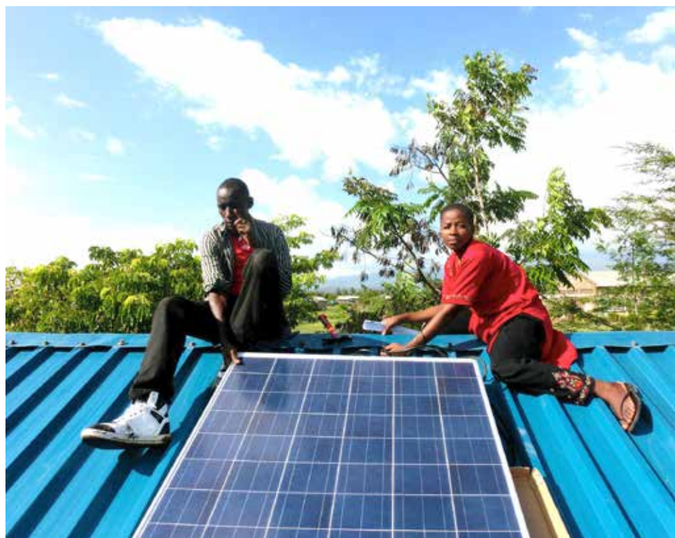
Solar Home Systems in Tanzania
